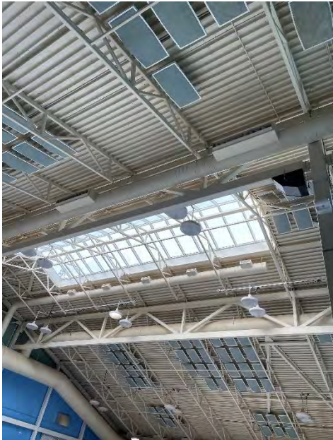
Photo 13 – Pool HID Lighting
