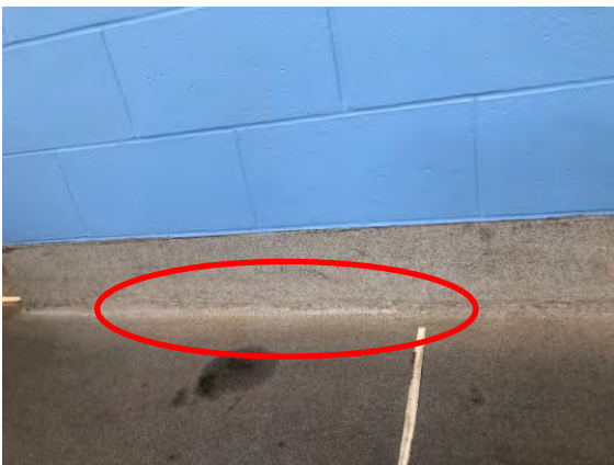
Photo 17 Crack at base of wall
