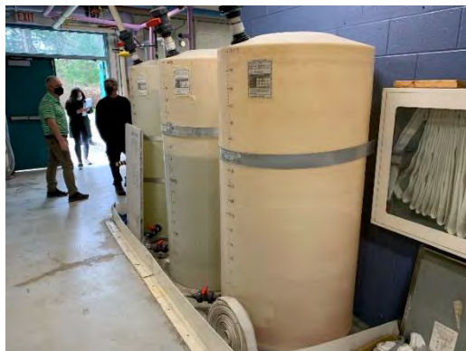
Main Chemical Tanks
