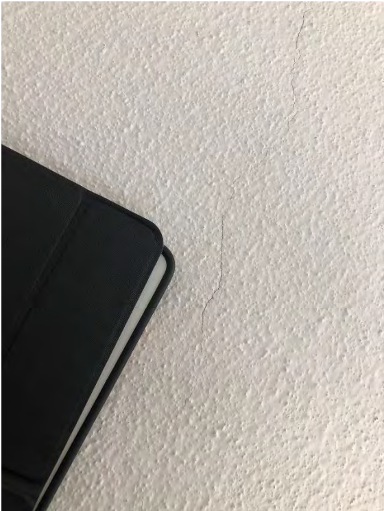
Photo 9 Close-up of crack in Photo 8
