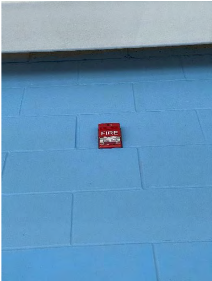
Photo 29 - Fire Alarm Strobe
