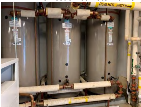
Domestic Hot Water Tanks
