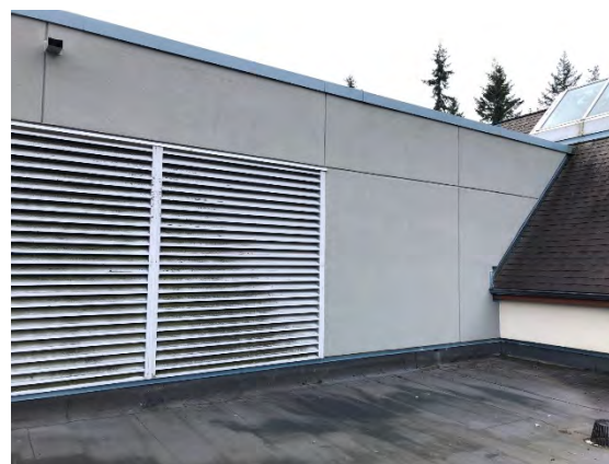
Photo 20 Vent at roof mechanical wall
