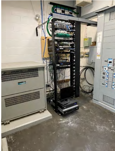
Photo 30 – Main incoming Telus/Shaw Demarcation
