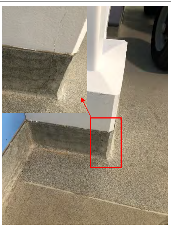
Photo 20 Crack at column base
