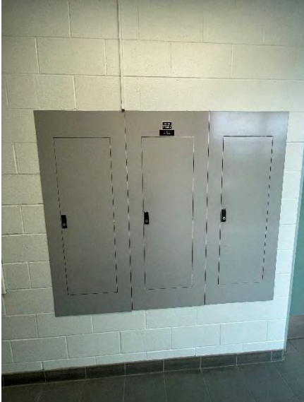
Photo 6 – Typical 208Y/120V Panelboard
