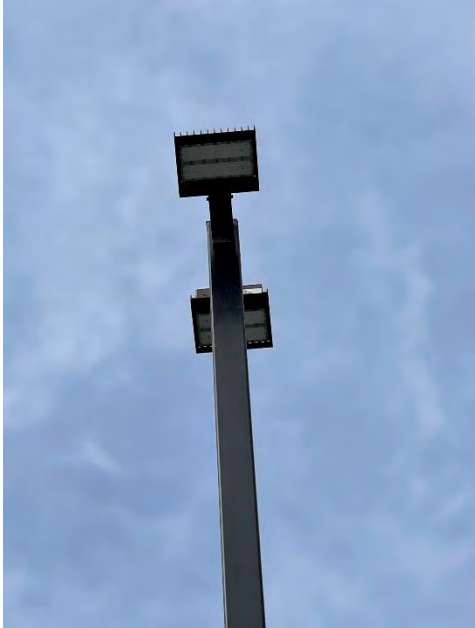
Photo 10 – Exterior Parking Lot lighting
