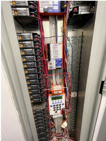
Photo 7 – Lighting Control Panel
