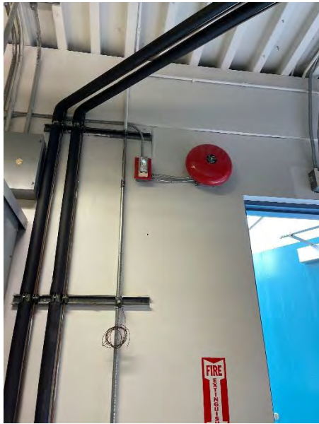
Photo 27 – Fire Alarm Bell
