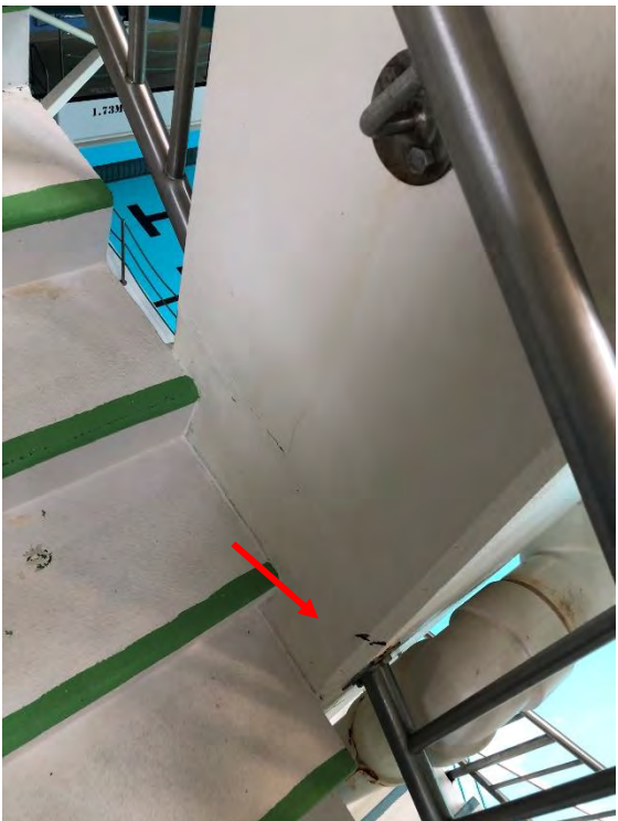
Photo 16 Damage/deterioration of column
