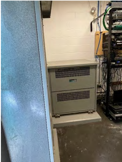
Photo 3 – 600V – 120/208V Transformer
