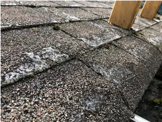
Photo 14 Exposed fiberglass core on shingles
