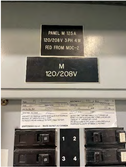
Photo 5 – Typical 120/208V Panelboard
