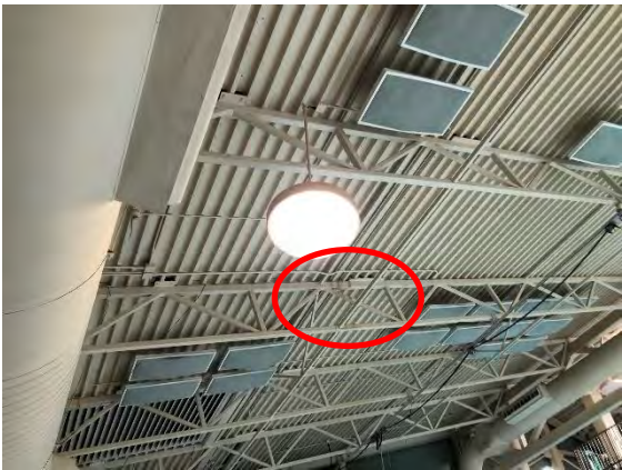
Photo 12 Staining on roof truss
