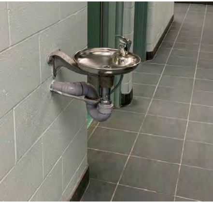
Photo A12 Drinking Fountain at Corridor 135
