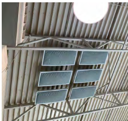
Photo A5 Suspended Acoustic Panels at Natatorium
