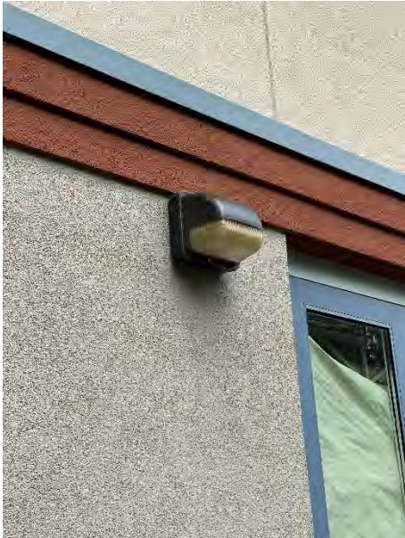
Photo 11 – Building Wall Mounted Lights
