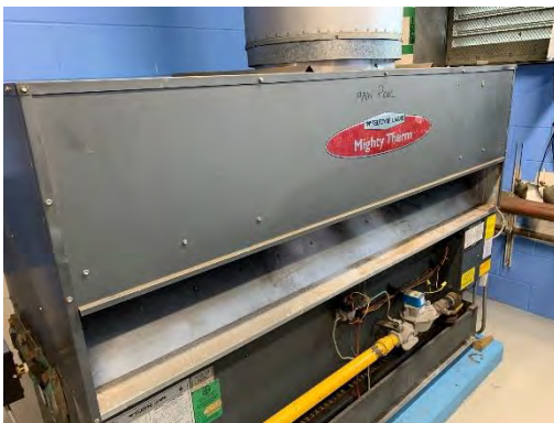
Main Pool Heater
