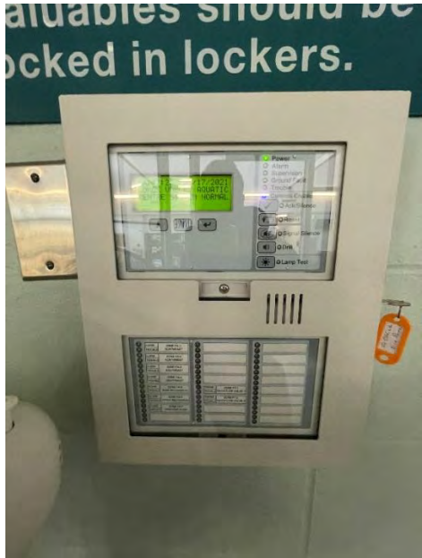
Photo 24 –Fire Alarm Annunciator
