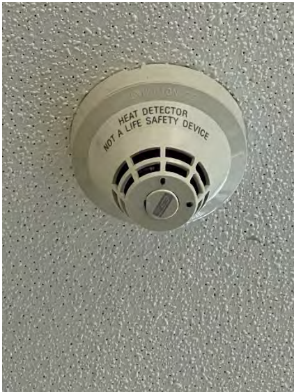
Photo 28 - Fire Alarm Heat Detector
