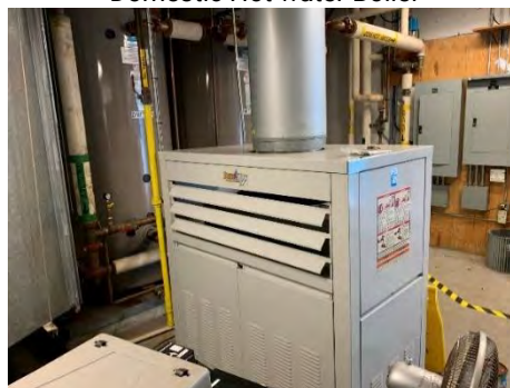
Domestic Hot water Boiler
