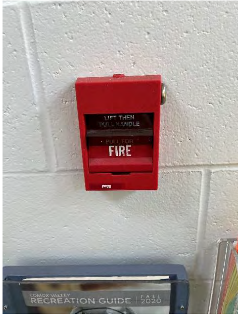
Photo 26 – Fire Alarm Manual Station
