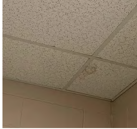
Photo A11 Staining at acoustic ceiling tile at Rm. 138 (Concession).
