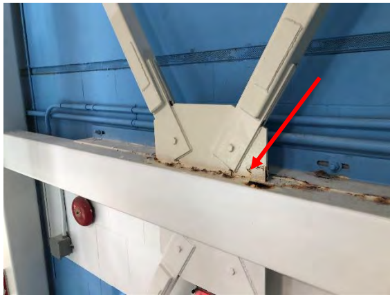
Photo 14 Corrosion at steel bracing
