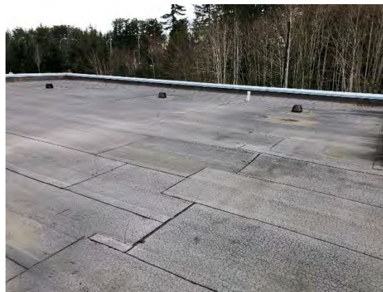
Photo 16 Ageing roof membrane at flat roof
