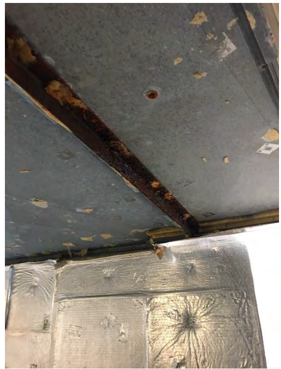
Photo 23 Corroded duct support
