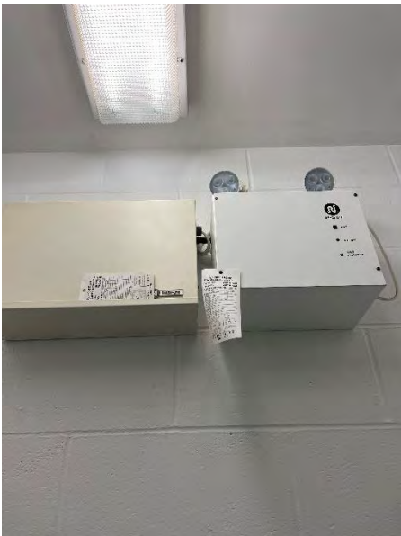
Photo 11 – Emergency Lighting/Battery Pack
