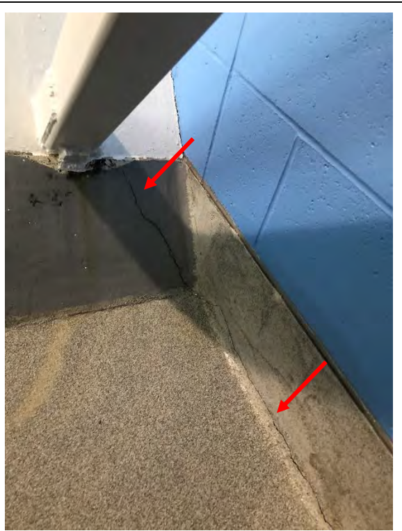
Photo 19 Cracked concrete at brace
