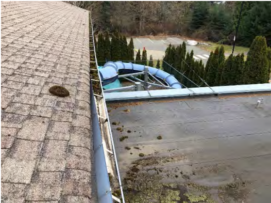
Photo 15 Damaged gutter on south elevation
