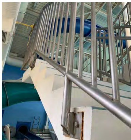
Photo A6 Stainless steel guards at pool
