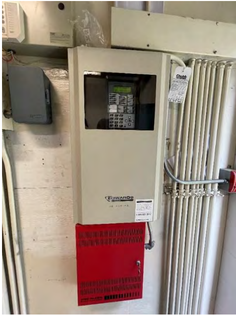
Photo 25 – Fire Alarm Control Panel
