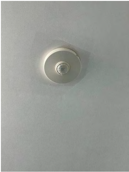
Photo 8 – Washroom Occupancy Sensor
