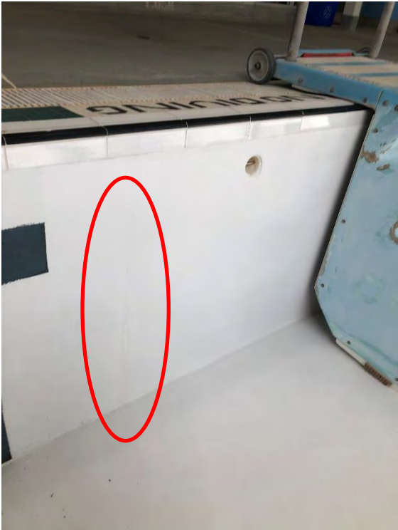
Photo 10 Crack in wall of pool at south end
