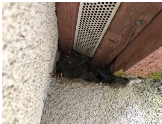
Photo 17 Gap in EIFS membrane at fascia detail
