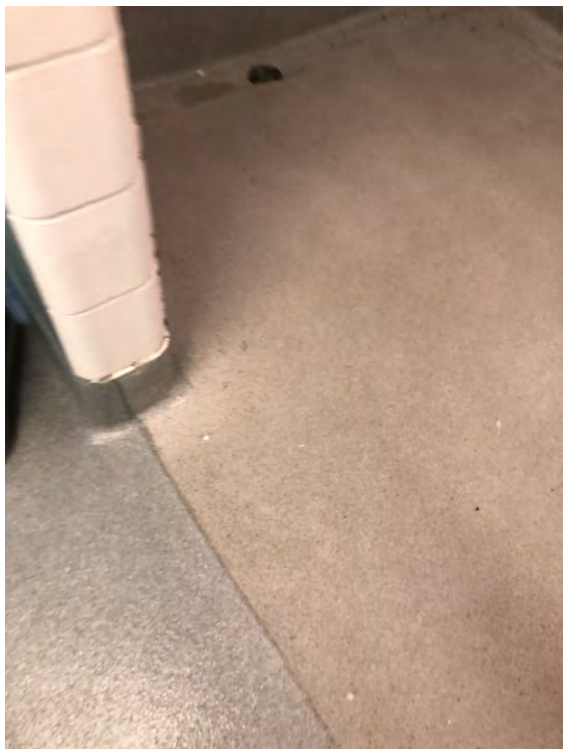
Photo 7 Joint in coating at changeroom
