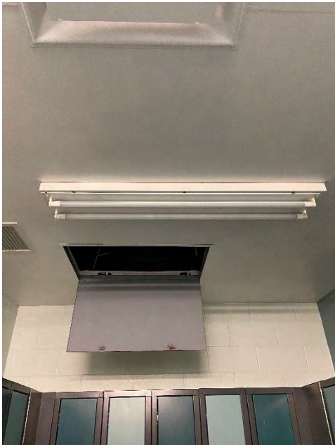
Photo 14 – Changing Room Lighting
