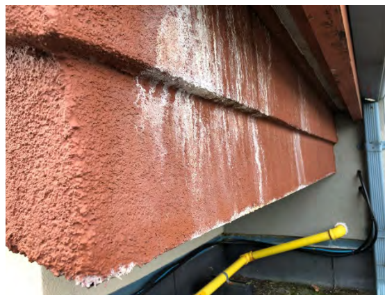
Photo 18 Efflorescence at roof eave (at gutter locations)
