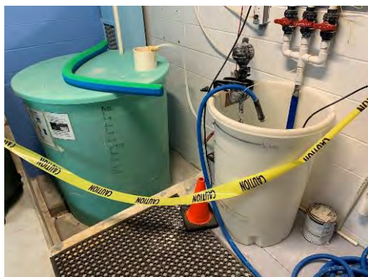
Bulkfeed tank w/Agitator & Sodium Hypochlorite
