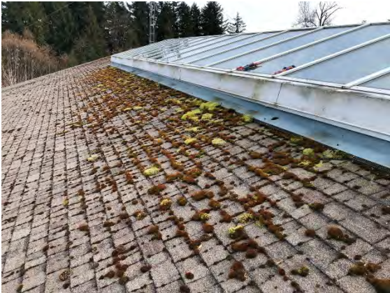
Photo 13 Organic growth at section of roof
