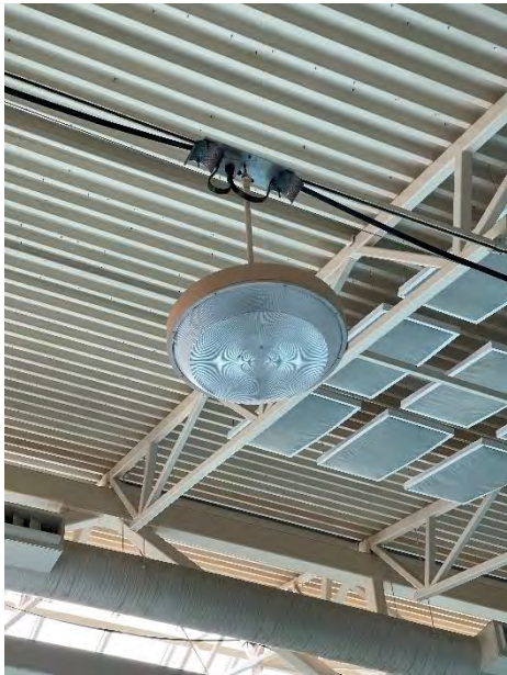
Photo 12 – Pool HID Lighting
