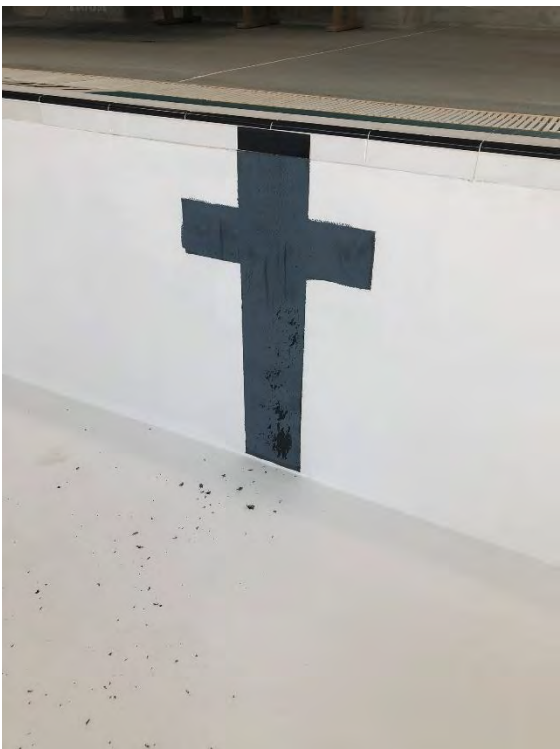
Photo 11 Flaking paint markings
